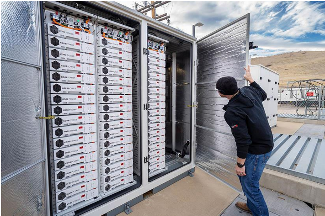
Plate 1-5: BESS access from the outside (Source: NREL)
